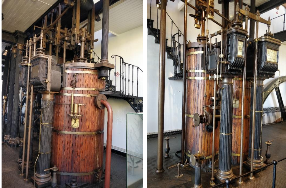
Windsor Steam Engines in the Barbadinhos Pumping Station
